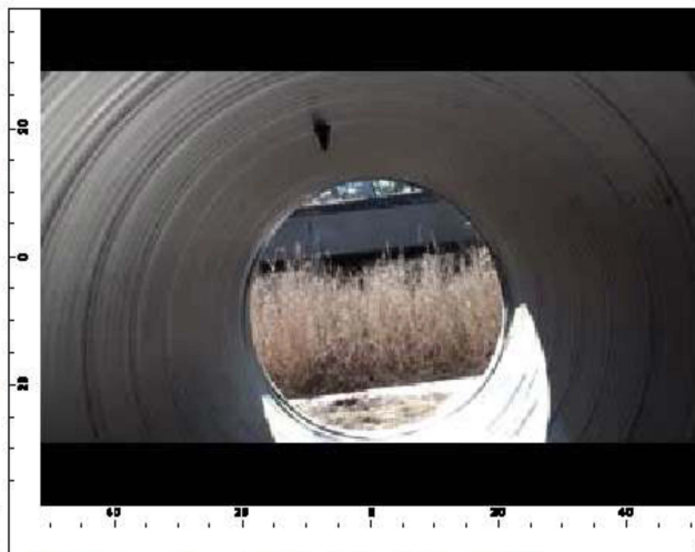
Stake for erosion control driven through crown of pipe.
