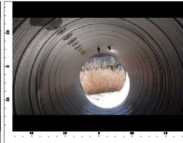
Slight dent at left springline at 78 ft.
