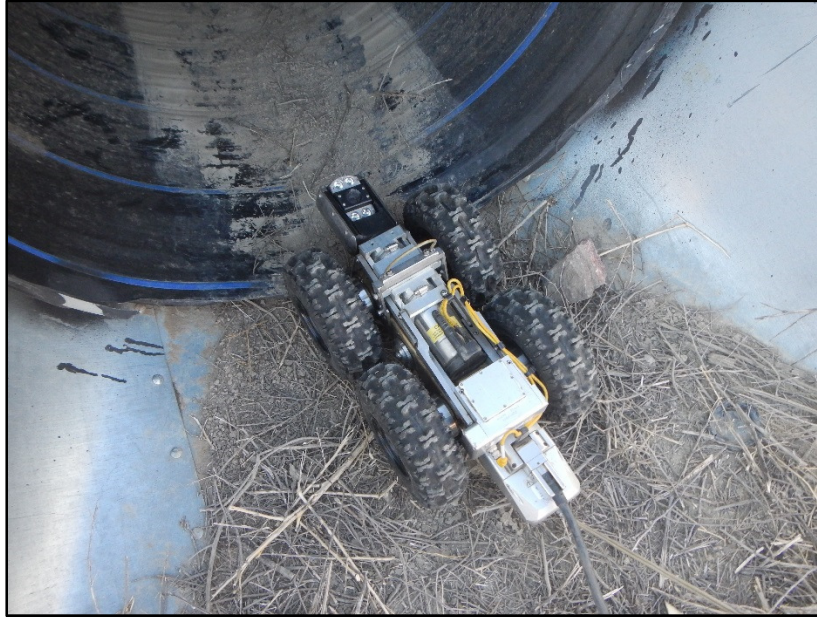
Figure 35. Motorized robot carrying CCTV entering HDPE pipe near Colorado Springs, CDOT Region 2
