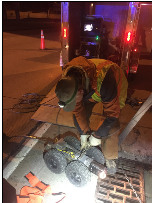
Figure 3610. Motorized robot carrying CCTV entering HDPE pipe along T-Rex Project site on I-25
