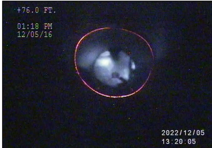
Figure 43. Typical laser ring projected onto the internal surface of failed pipe
