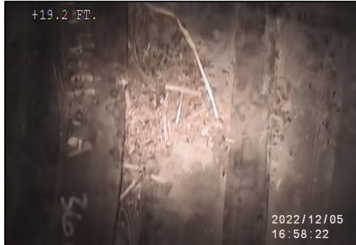
Figure 55. Close-up of a separated joint using CCTV recording
