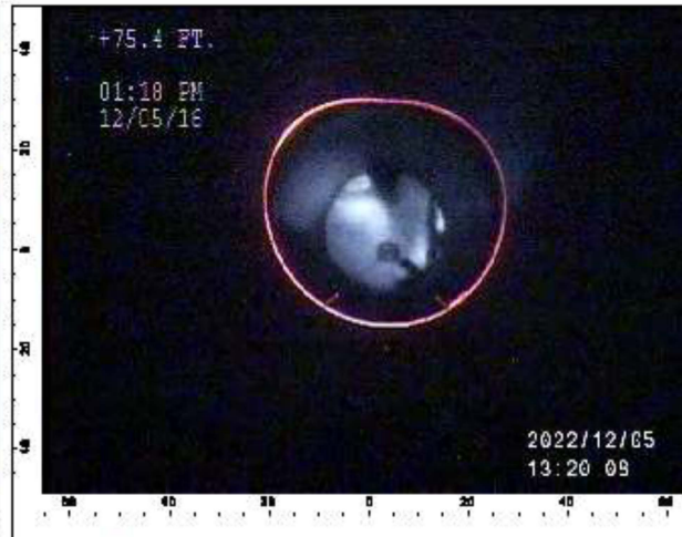
Pipe deflected approximately 5.8%.
