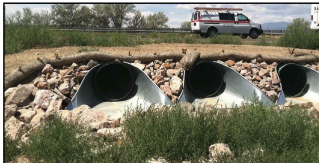
Figure 5. HDPE pipes with metal outlets across Interstate 25
