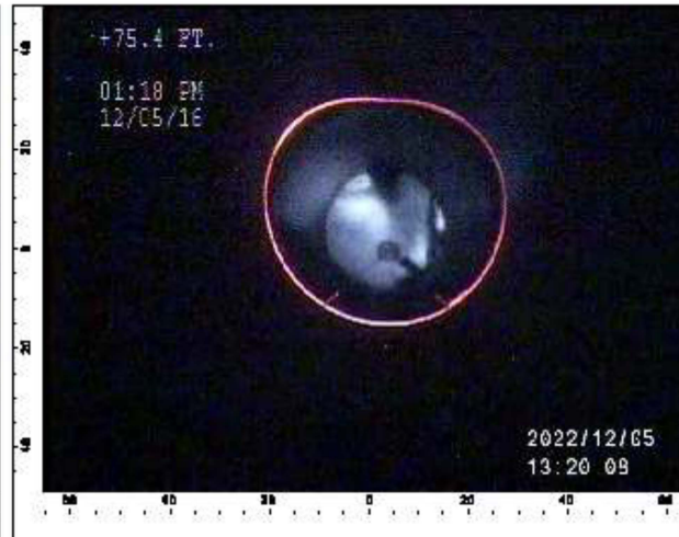
Pipe deflected approximately 5.8%.
