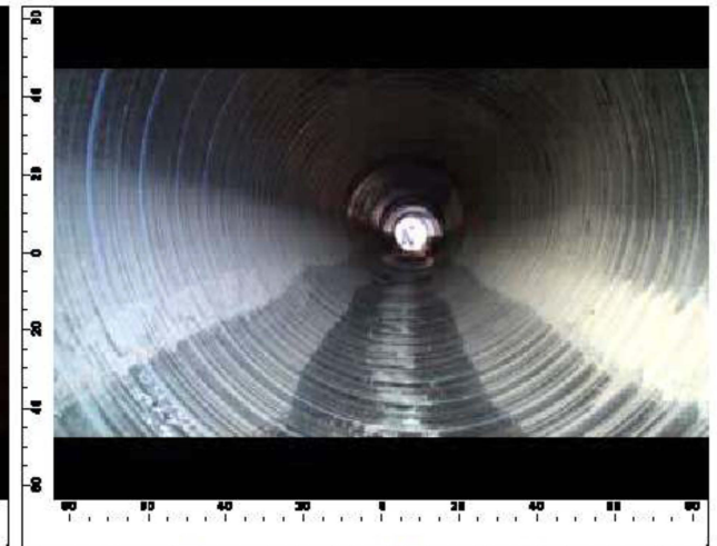
View from outlet end, pipe slight racked near outlet end not caught by laser.
